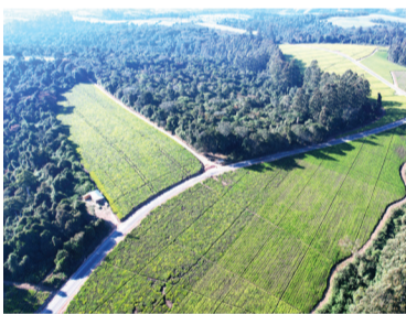
The 30.3 kms of tarmac road extending from Sawala - Mkonge - Iyegeya in Mufindi district, Iringa region. The road is part of the 311 kms of road networks under construction through AGRI-CONNECT programme aiming to facilitate easy access to market for agricultural produces.
