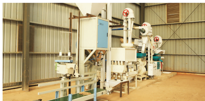
Inside the GGML funded Saragurwa Rice Paddy Project storage and processing unit.
